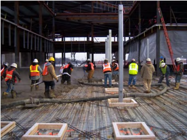
WELDED WIRE FABRIC: CLUTTERED DECK WITH EXTENSIVE TRIP HAZARDS, MESH OUT OF POSITION RESTING ON TOP OF DECK
