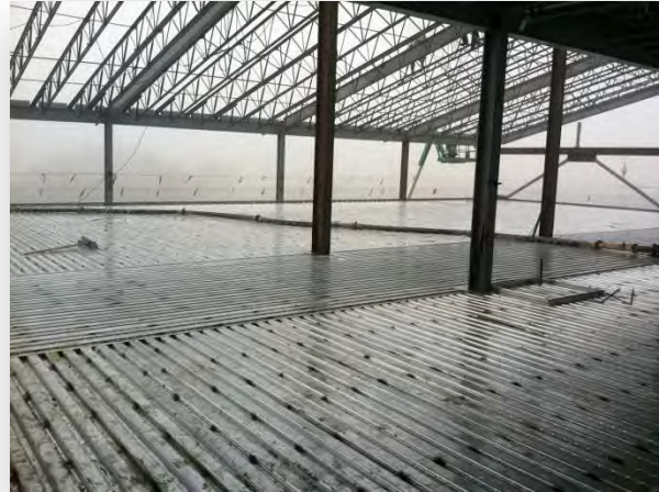
WITH CFS 150-5: A CLEAN DECK FREE FROM TRIP HAZARDS
