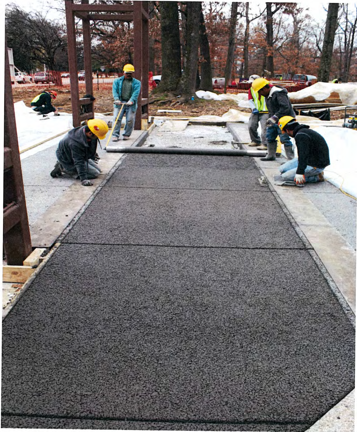
The terrace itself is largely pervious concrete with a charcoal gray integral pigment. This large area is shouldered by three variously sized “sprockets”, all of which are encompassed by a perimeter “chain” calling to mind the gears and workings of a bike.
